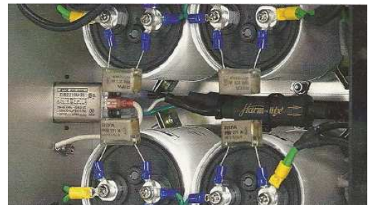
Harmonix on the outside and an Enacom line filter on the inside
